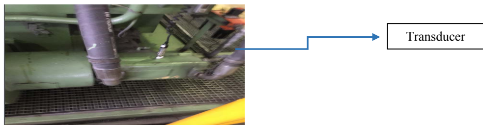
Fig. 5 – Accelerometer (transducer) position on the pump machine.
